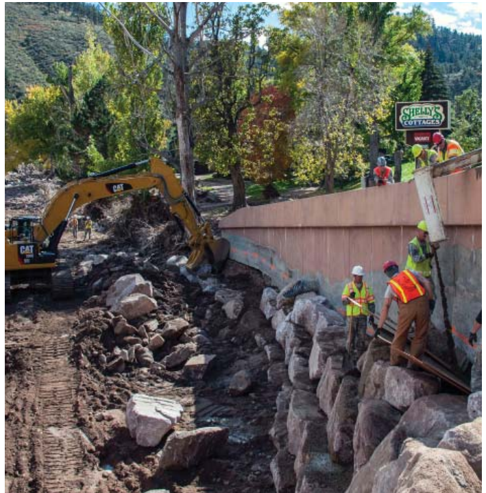
Members of the 219th RED HORSE Squadron of the Montana Air National Guard build a retaining wall for the North Saint Vrain Creek on Oct 21, 2013. The unit deployed to Colorado to assist in flood relief efforts. National Guard photo by Senior Master Sgt. John Rohrer.
